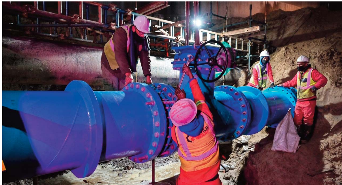
Bulking up water infrastructure: In August, the City's Water and Sanitation team completed the complex upgrade of the 700 mm bulk water supply line feeding the Blaauwberg area in less than 24 hours. The work was necessary to improve the reliability of water supply to the area.
