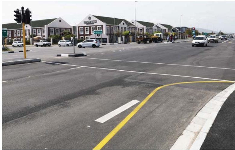
Beating the Bosmansdam bottlenecks: The upgrade of Bosmansdam Road between Koeberg Road and Montague Drive, which started in November 2019, is now complete.
